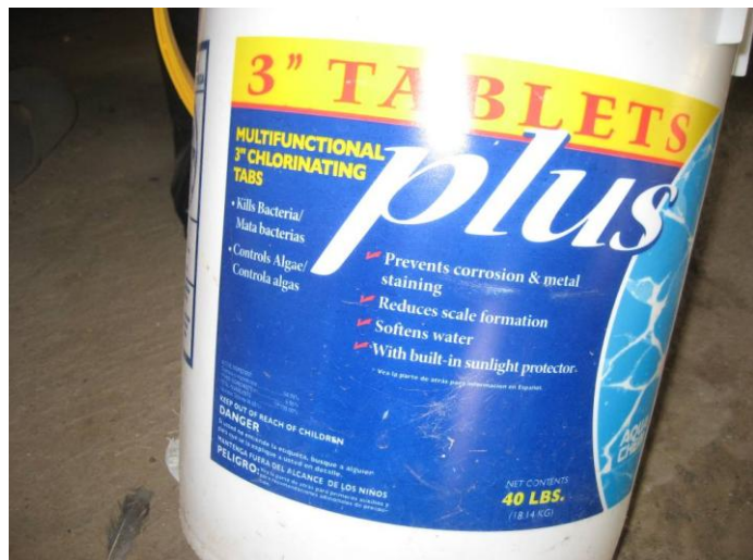
Chlorinated tablets used in conjunction with the residence’s water pump that distributes well water to the home.
