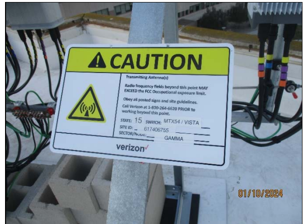
40. Verizon Sector C Caution Sign Close Up
