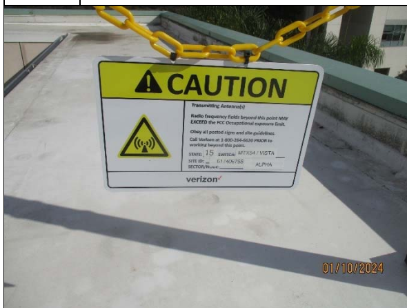
15. Verizon Sector A Barrier Caution Sign Close Up
