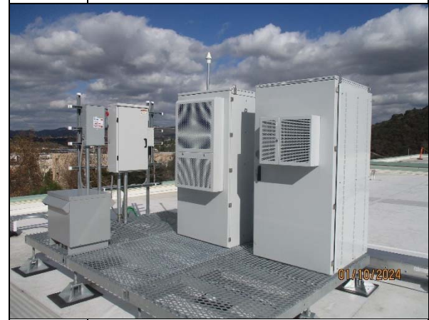
5. Verizon Equipment- No RF Signage
