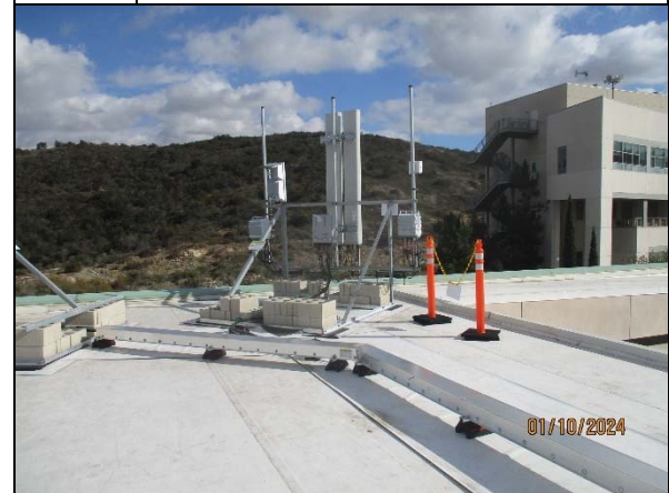
6. Verizon Sector A Overview
