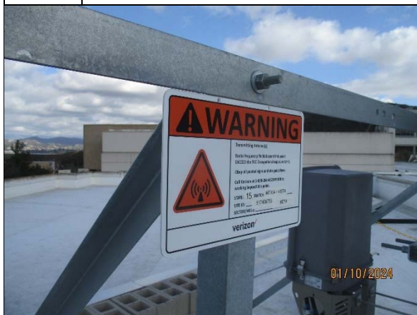
26. Verizon Sector B Warning Sign
