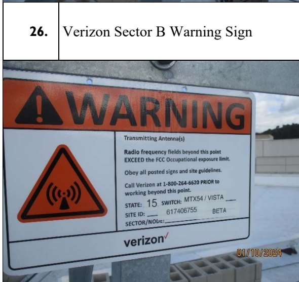
27. Verizon Sector B Warning Sign Close Up
