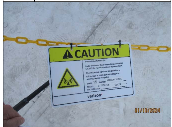
48. Verizon Sector D 14' Barrier w/ Caution Sign Close Up
