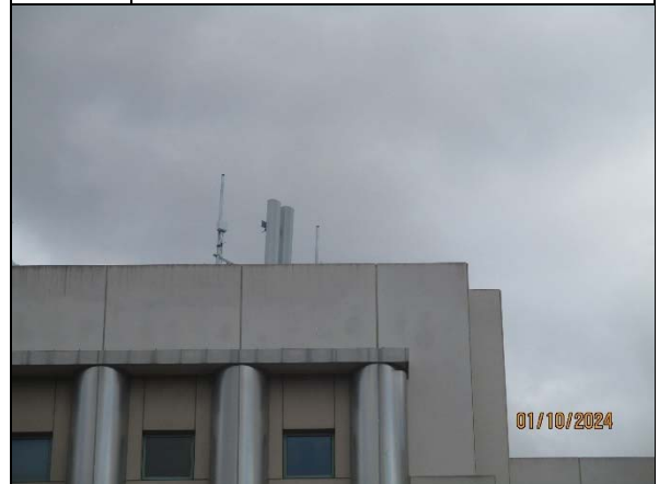
36. Verizon Sector B Ground View Close Up
