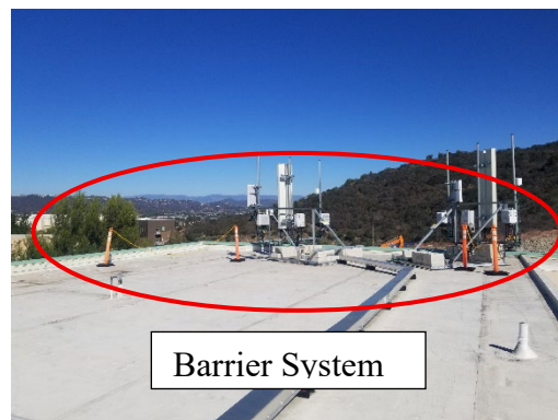
Image 4: Northeast Corner Array
