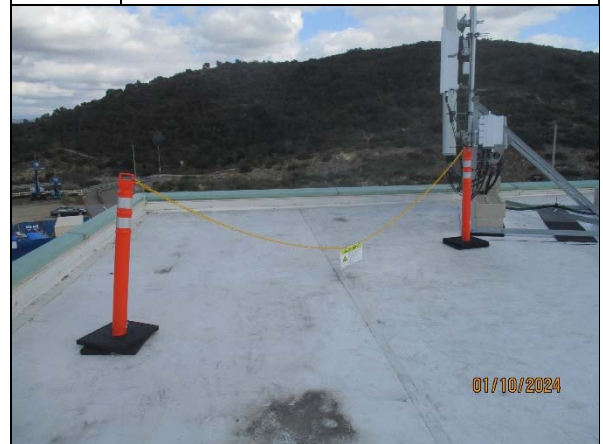
47. Verizon Sector D 14' Barrier w/ Caution Sign
