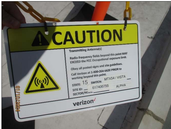
13. Verizon Sector A Barrier Caution Sign Close Up
