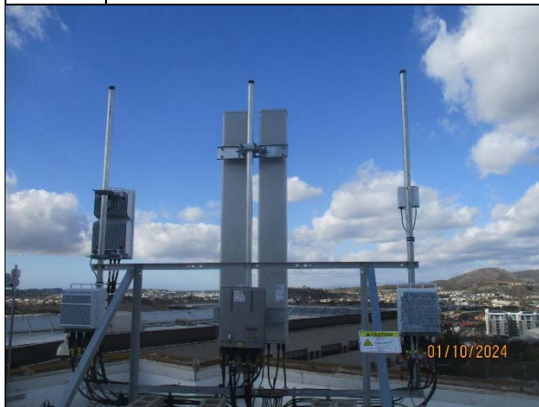
38. Verizon Sector C Antennas
