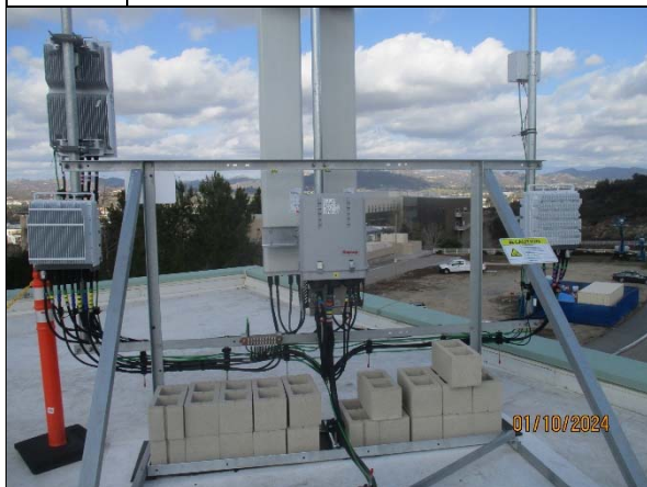
45. Verizon Sector D Caution Sign
