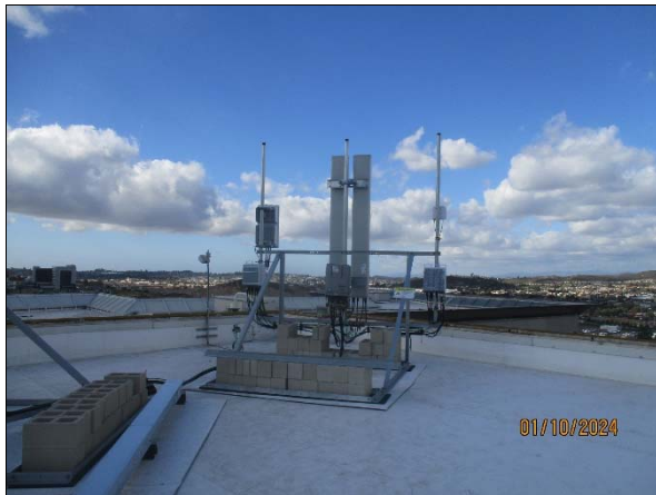
37. Verizon Sector C Overview
