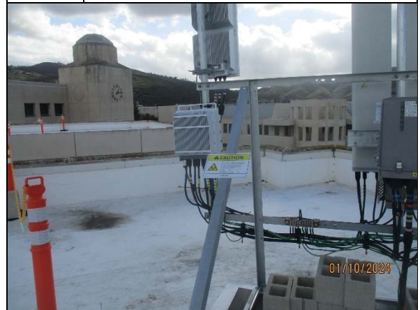
24. Verizon Sector B Caution Sign
