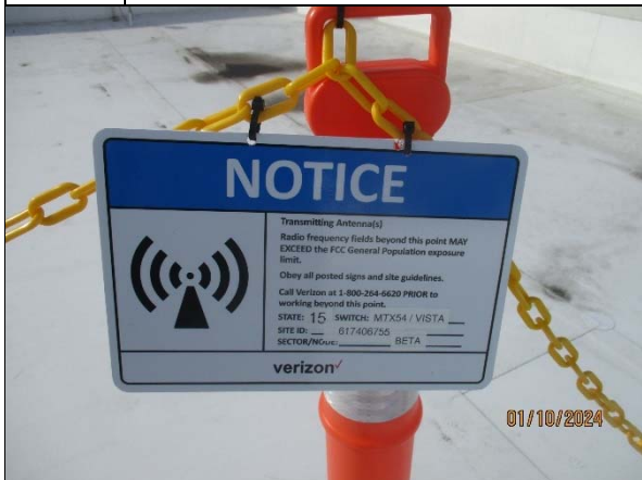
33. Verizon Sector B 38' Barrier w/ Notice Sign Close Up
