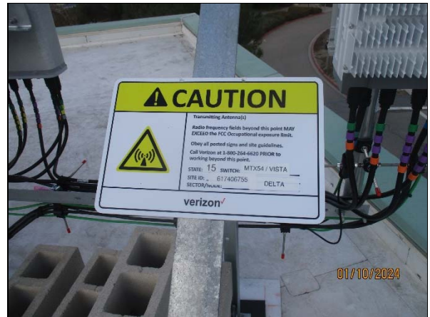
46. Verizon Sector D Caution Sign Close Up
