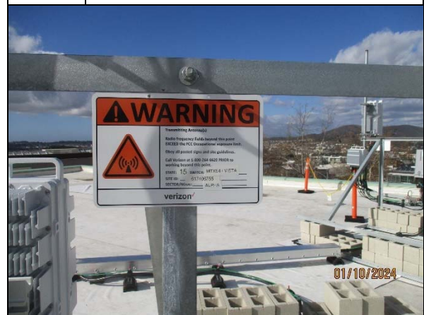
17. Verizon Sector A Barrier Warning Sign Close Up
