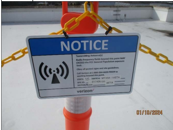
32. Verizon Sector B 38' Barrier w/ Notice Sign Close Up
