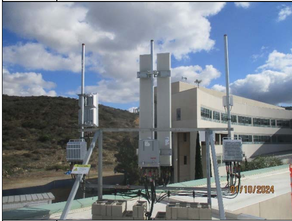
8. Verizon Sector A Antennas
