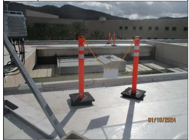
11. Verizon Sector A 4' Barrier
