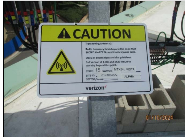
10. Verizon Sector A Caution Sign Close Up
