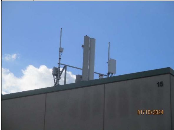
50. Verizon Sector D Ground View Close up
