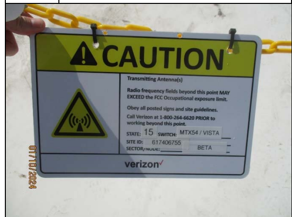
29. Verizon Sector B Barrier Caution Sign Close Up
